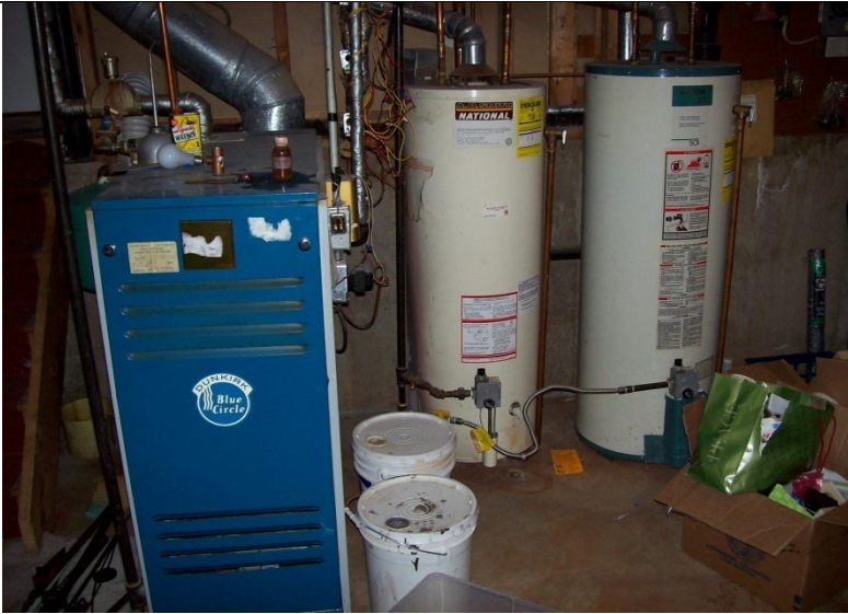
This image shows a 65% efficient boiler next to 2 water heaters in a 2300 sq/ft home. This all could be accomplished with a single 90%+ efficient boiler.
