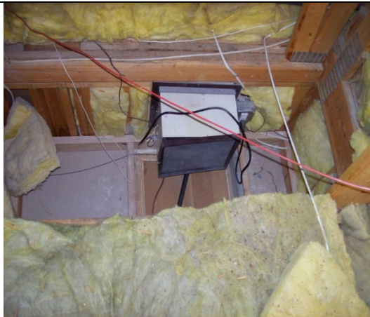
This humidifier is open to the attic and blows cold damp air laced with fiber glass into the home.
